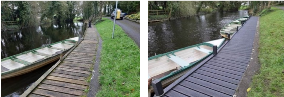
Images: The old timber on Finea Bridge was removed (left) and replaced with composite timber in a similar style (right).
