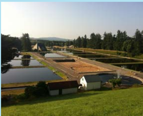
Vartry Water Treatment Plant. Photo: Nicholas O'Dwyer.
